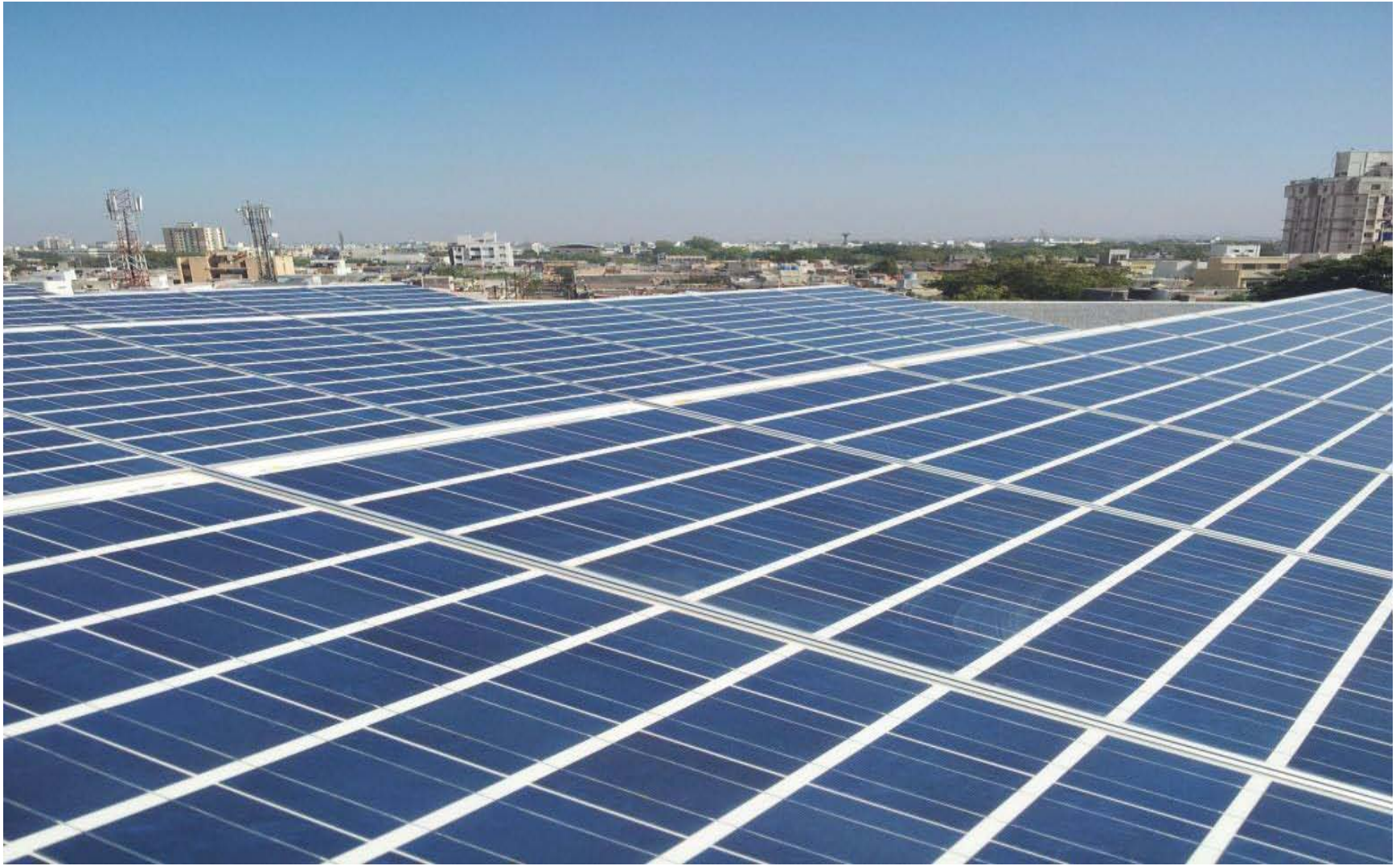
1 MW solar PV Roof-top project in Delhi
